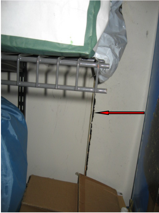
The side rear garage wall has visible daylight at this unsealed gap between the concrete and framed sections of wall.
