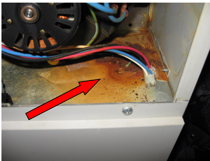
The interior of the furnace exhibits unusually heavy corrosion, given the age of the unit. (about 4 years old)
