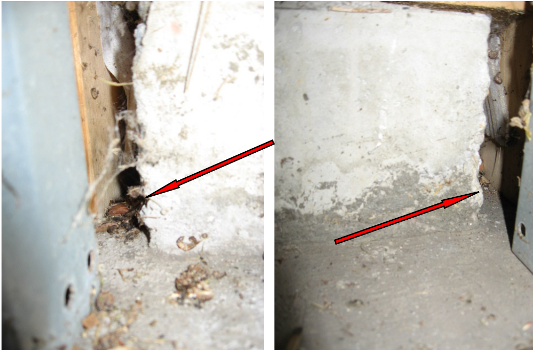
These gaps beside each garage door should be sealed to prevent water, insect and vermin intrusion.
