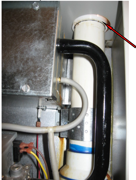
The indicated area was wet and there was no evidence of PVC cement at the coupling.
